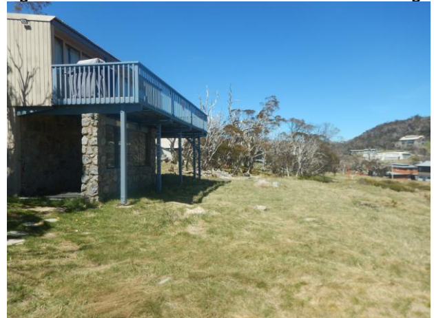
Figure 8: Photo of the western elevation of the lodge and the deck to be replaced
