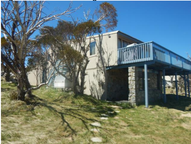
Figure 7: Photo of the western and northern elevation of the lodge and the deck to be replaced
